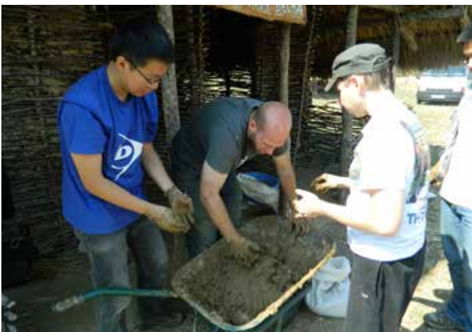
The UCL team is mixing the local clay with river sand and organic matter for lining the installations.
