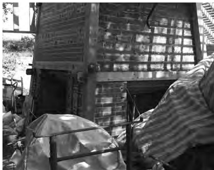
Photograph of the blast furnace taken during the construction of the new cover building.
