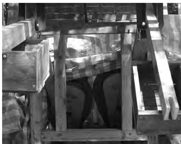
Photograph of the bellows taken during the construction of the new cover building; the new build means that the bellows and other parts of the furnace are protected by tarpaulin.
