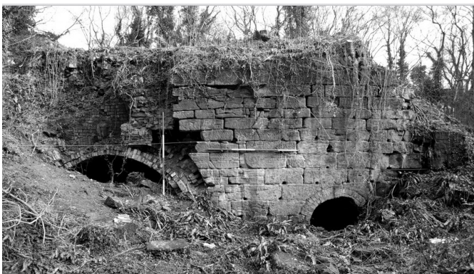
Figure One Fig. 1. Stirchley furnaces: view of part of the western elevation before excavation, showing the top of the arch of the northern furnace and the smaller archway of a passage between the two furnaces. The ground level here is approximately 2.5m above the original floor levels. Photo: Paul Belford/Nexus Heritage.
