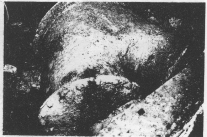
D Y-junction in turbine feed pipe at Lower Wireworks site; right-hand branch feeds turbine, left-hand branch blanked off.
