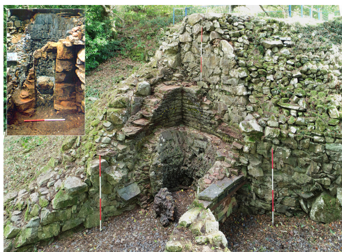
Fig. 1. A perspective view from a height of about 4m, looking over the furnace pillar, with the blowing arch on the left and the tapping arch on the right. Scale rods 2m. Inset: Detail of the tapping arch excavated in 1984. The tapered opening in the sandstone blocks, which would be blocked during use, gave access to the crucible for repairs to the lining. Scale rod 1m
